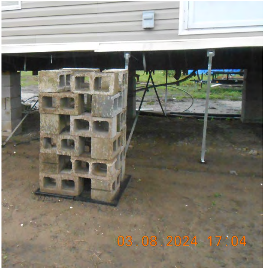
C2.e) Lowest machinery serving building is AC located near rear center of home.
